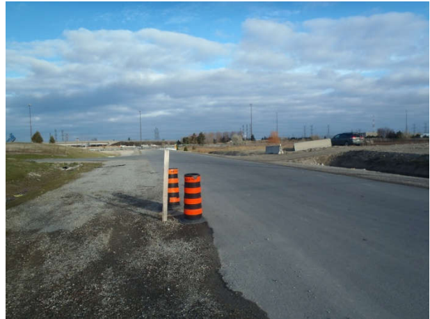
Plate 74 [N]: Newly paved access road and staging area (right) for the 407 ETR Concession Company Ltd.; no potential
