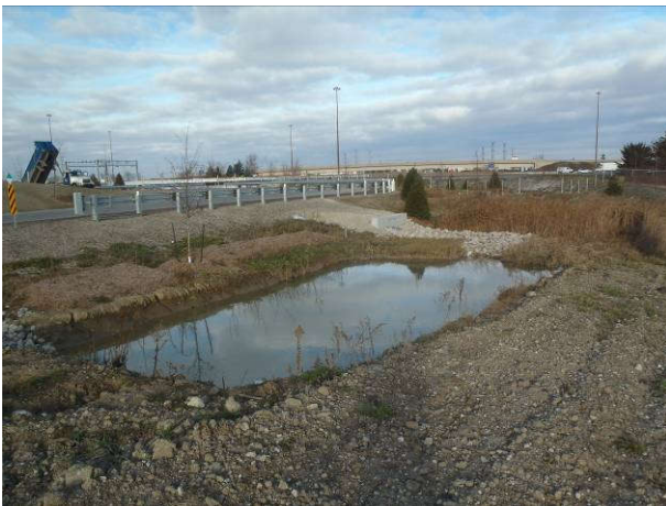
Plate 75 [NW]: Newly installed drainage culvert as part of 407 ETR Concession Company Ltd.; no potential
