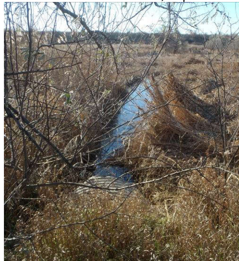
Plate 94 [SW]: Permanently low and wet tributary of the Lower Humber River; no potential (note: culvert is for overlying hydro corridor gravel access road)
